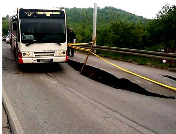
Main road M18, Banj Brdo, Priboj – Simin han km 14+420 – 14+650, Landslide above and below road grade line (Flods 2014)
